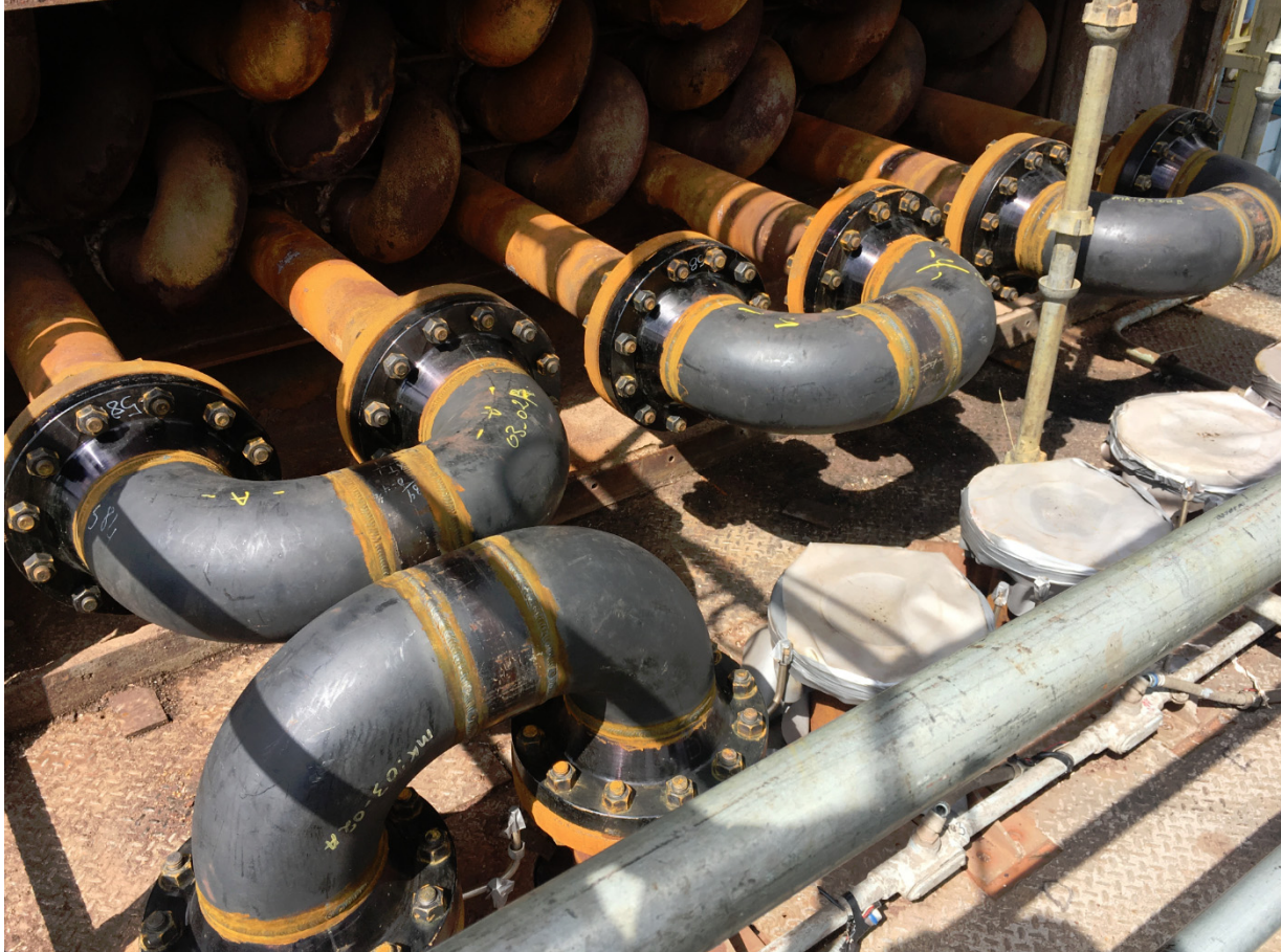
Figure 8: Tubes Looped at Top of Radiant Section
